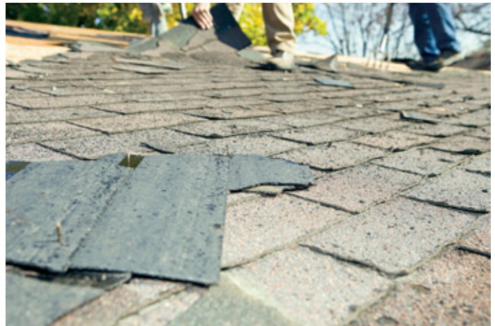
Hail-damaged asphalt shingle roof.
